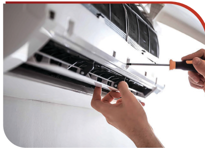
AIR CONDITION SERVICE
